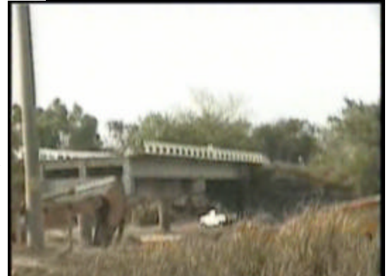
The bridge to Enolia (sp?) and Santa Maria was washed out in the hurricanes.
